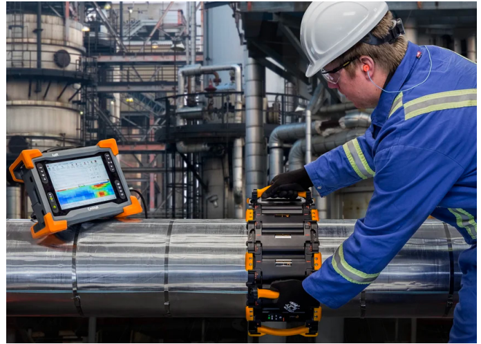
Figure 4: Lyft PECA pipeline CUI.
